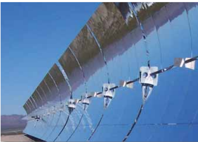
Parabolic trough systems are considered the most reliable and least costly of today's solar-thermal electricity (STE) technologies. The Nevada Solar One plant—a 64-MW installation that lines up 760 parabolic concentrator arrays—began generating power in June. (photo: Acciona Group)
