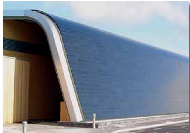
Thin-film photovoltaic cells, manufactured by depositing semiconductor materials on an inexpensive substrate, can be integrated with conventional building materials such as roofing tiles. In this 85-kW installation, CIS PV cells form an entire side of a business center in Wales. (photo: Shell Photographic Services, Shell International Ltd.)
